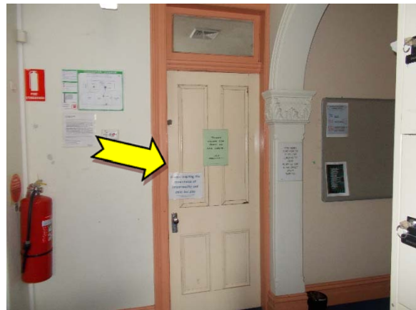
Photo 16. Interior, level one, throughout, skirting, window and door frames – lead-containing light orange upper paint systems.
