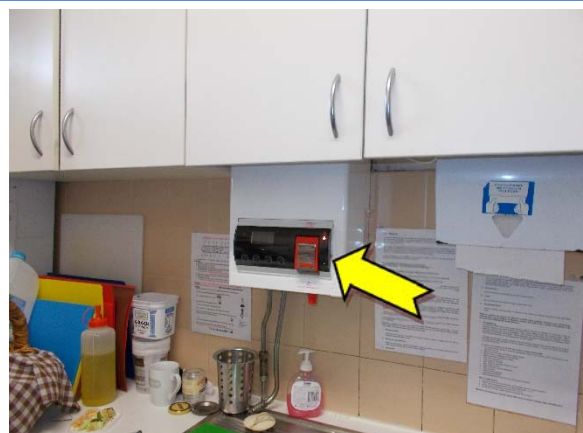
Photo 12. Interior, ground level, kitchen, hot water boiler – suspected SMF internal insulation material.
