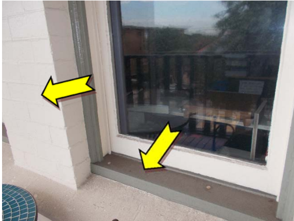
Photo 13. Exterior, level one, verandah, throughout, walls and window frames – suspected lead-containing cream and green upper coloured paint systems.
