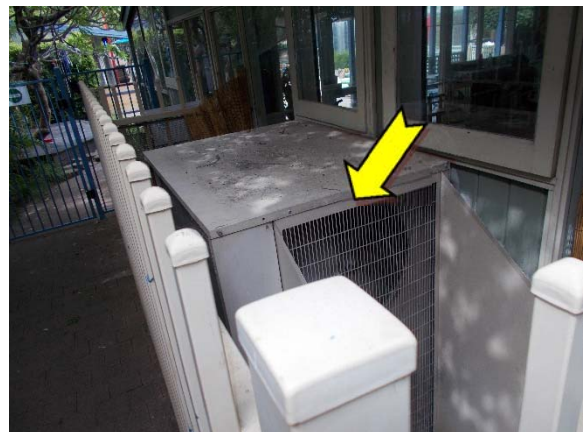
Photo 18. Exterior, ground level, east elevation, air conditioning unit – ODS-containing R22 refrigerant gas.
