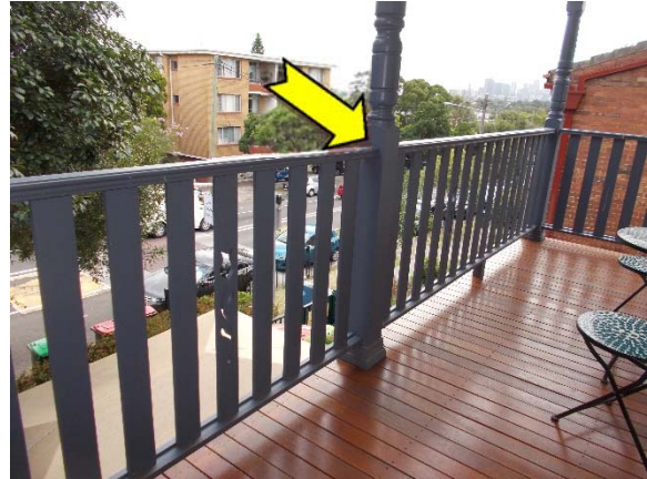
Photo 14. Exterior, level one, verandah, hand rails – suspected lead-containing blue upper coloured paint system.
