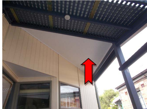
Photo 2. Exterior, ground level, south-west elevation, awning – suspected asbestos-containing fibre cement sheeting.
