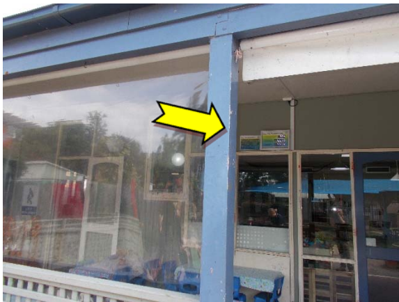
Photo 15. Exterior, ground level, throughout, frames and support – lead-containing cream lower paint system and suspected lead-containing blue upper paint system.
