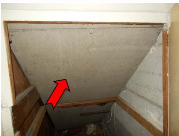
Photo 5. Interior, ground level, east elevation, under staircase – asbestos-containing fibre cement sheeting.
