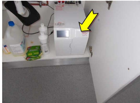
Photo 10. Interior, level one, kitchen, hot water boiler – suspected SMF internal insulation material.
